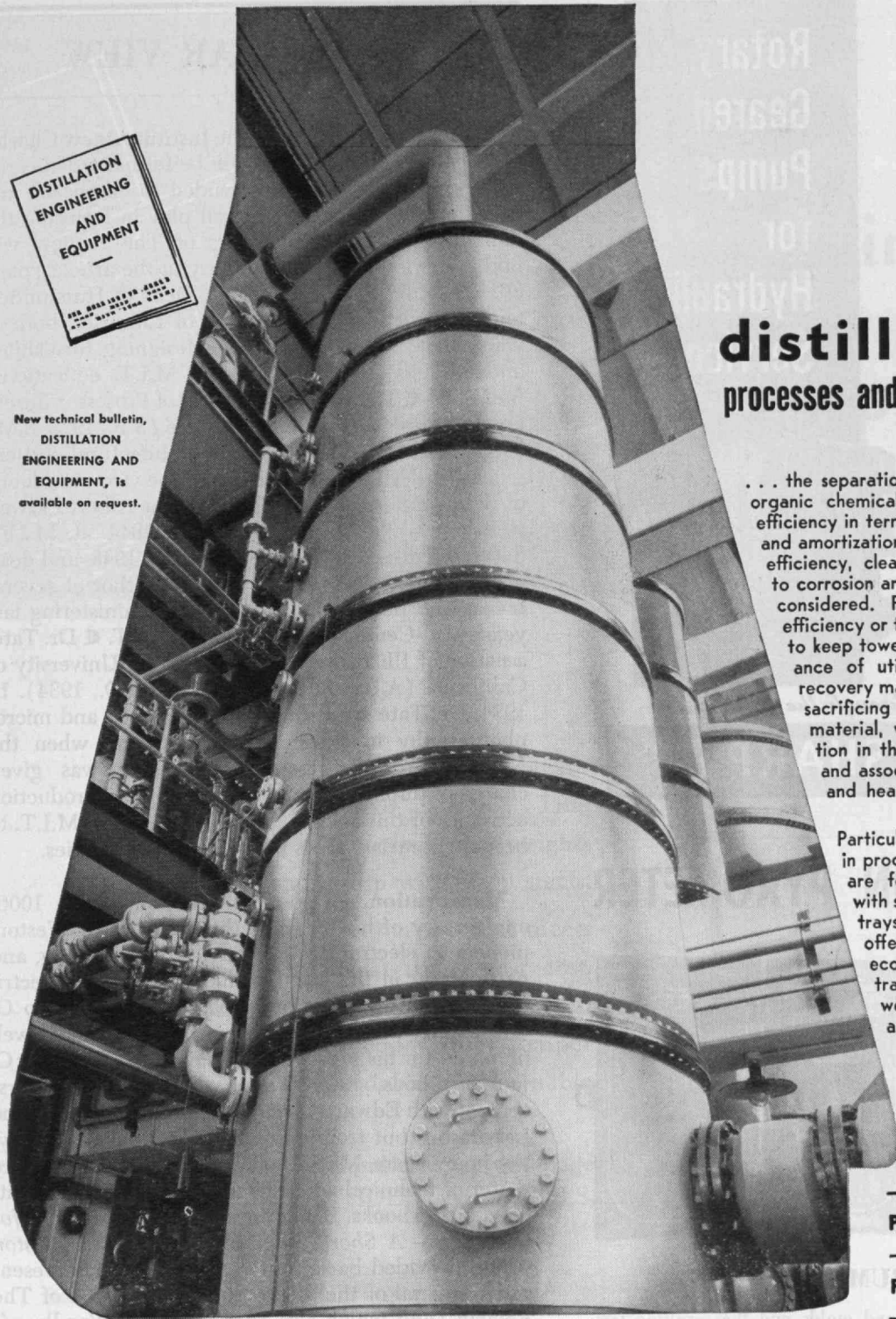
Distillation column of type 316 stainless steel measuring 56 feet in height, 10 1/2 feet in diameter, having six shell sections.
